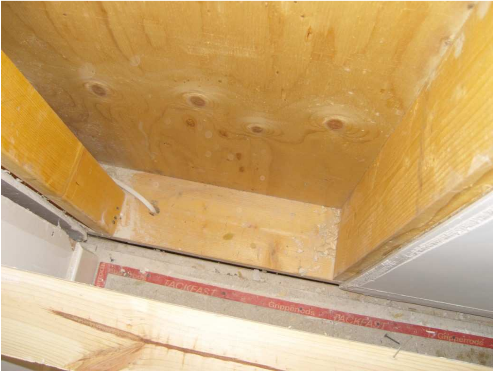
Outer Wall Not Fixed to 1st Floor Joist
