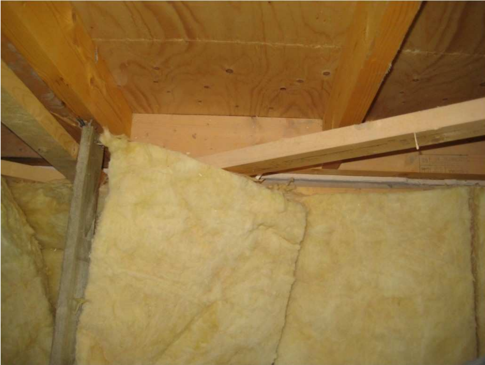
Spandrel Panel Not Tied Back to Roof Trusses
